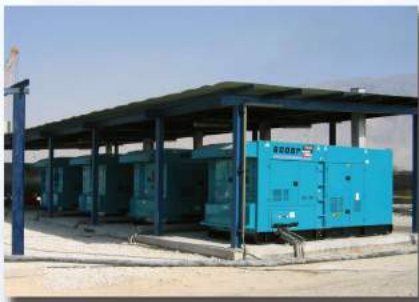
As the power source in the area where electricity is unavailable.
